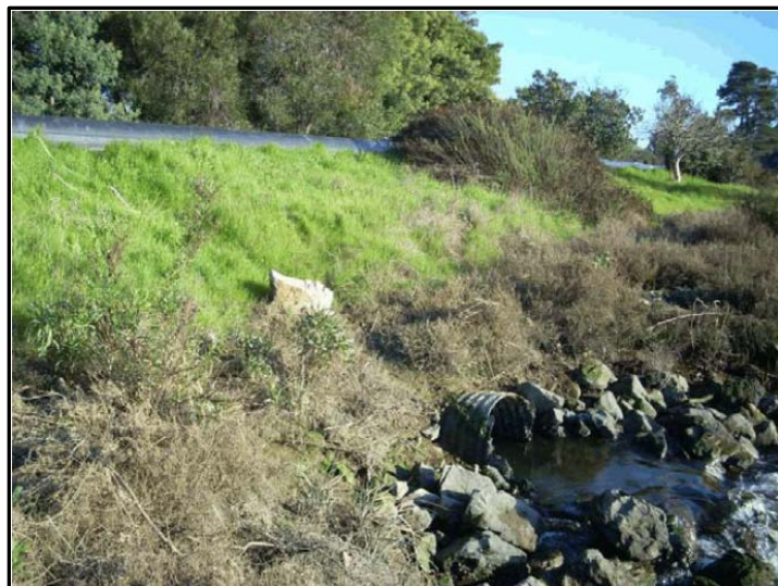
Old McAllister Slough culvert was heavily deteriorated
